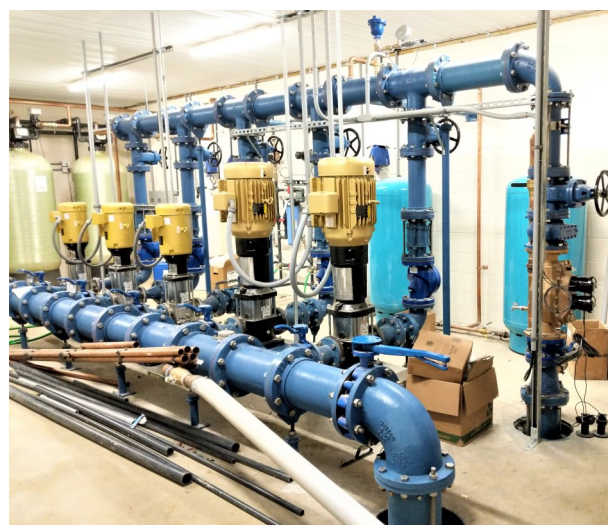
Newly constructed Wood Meadow 5 VFD pumping system, 0-500 gpm, in Windham, NH. The system was designed by Lewis Engineering, PLLC and is owned and operated by Pennichuck Water.
