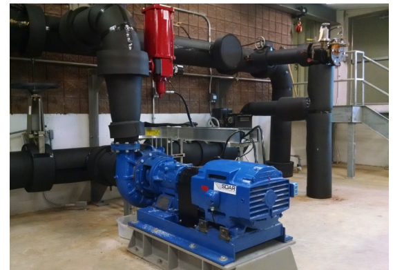
Berlin Water Works' energy recovery turbine at the Ammonoosuc Water Treatment Facility.
