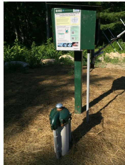
SDDW well at a maple sugar producer to provide water for operation of their facility and data collection platform for transmitting real-time water level and temperature data.
