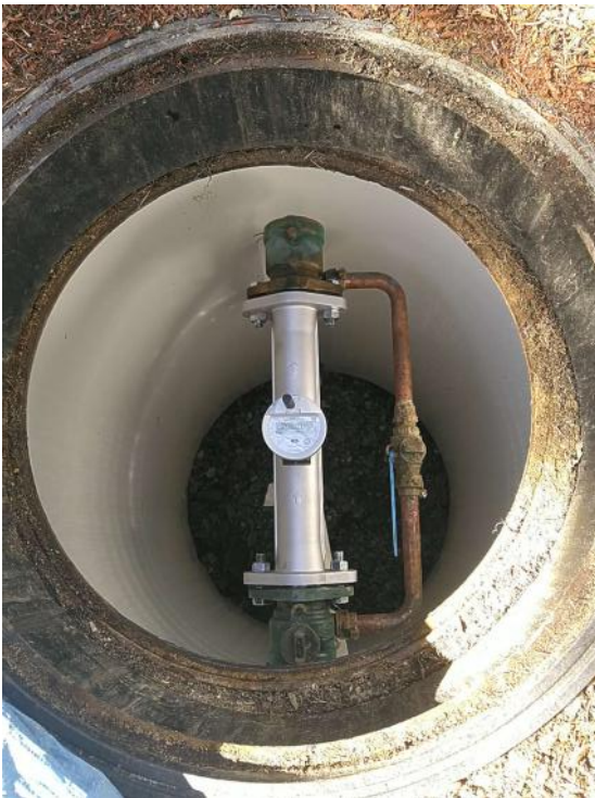
Meter location in a pit.
