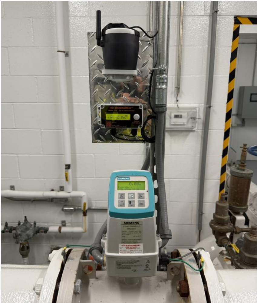
SCADA Metrics on well meter with AMI Radio.
