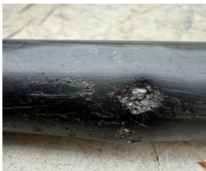
Damaged pipe from Aspen Lane leak.
