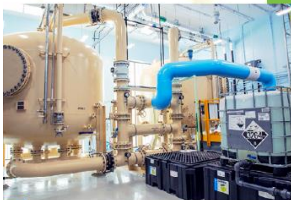
Grove Pond Water Treatment Plant, Ayer, MA (above). 1970s CDM Smith laboratory (below).
