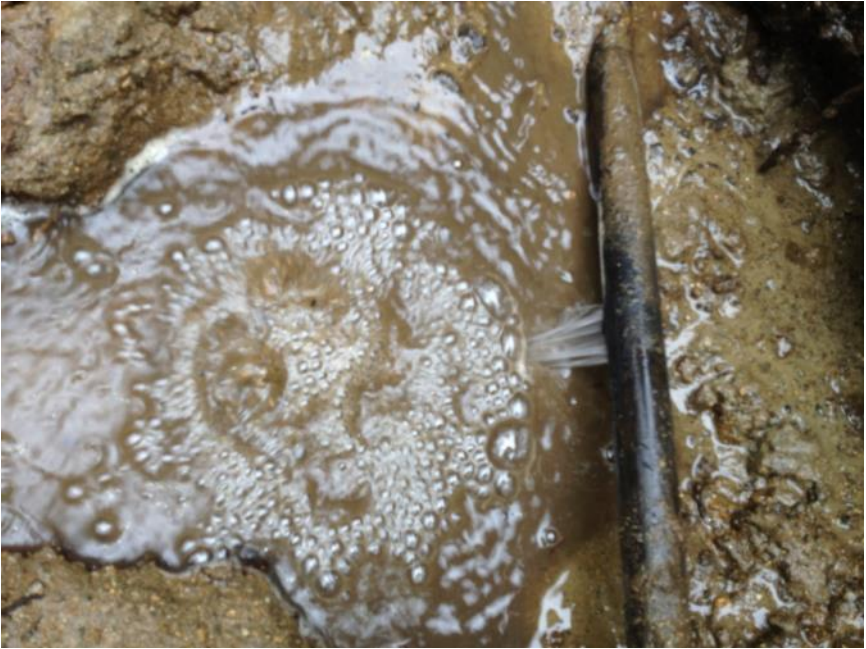
Plastic pipe with water exiting it through a break
