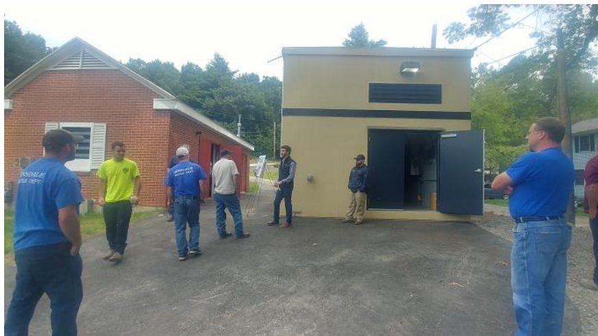
Above: The Oak Hill Pump Station's new structure to house electrical components. Below: New pump inside the original structure.
