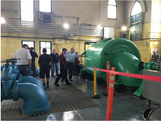
Inside the Cohas Avenue Pump Station.
