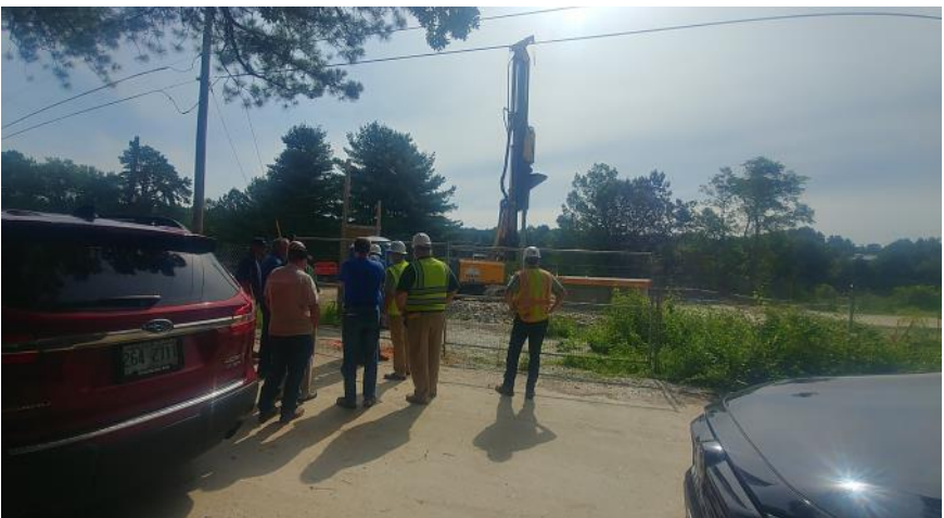
Location of Manchester Water Works' radial collector wells on the Merrimack River.
