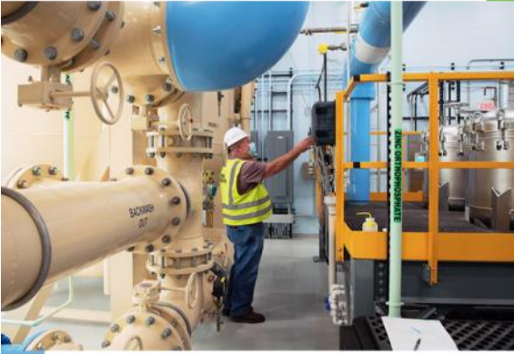
Grove Pond Water Treatment Plant, Ayer, MA
