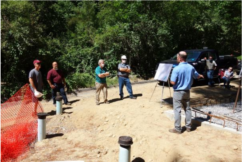
The Turkey Hill Booster Pump Station project was reviewed by Mike Metcalf, PE and Tim Puls, PE of Underwood Engineers, Inc.
