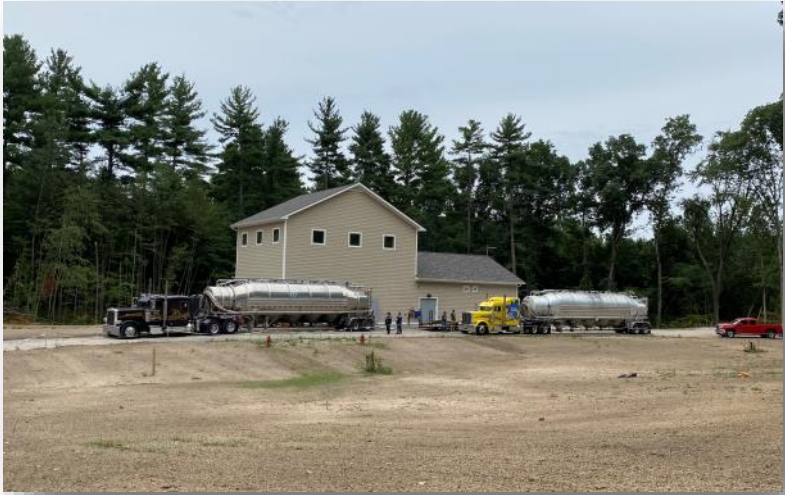
GAC tankers arrive at Merrimack Village District's Wells 4&5 new PFAS Water Treatment Plant.
