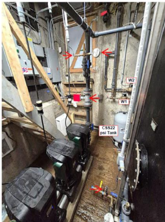
Atmos. Tank on Right, 3-DAB Pumps on Left
