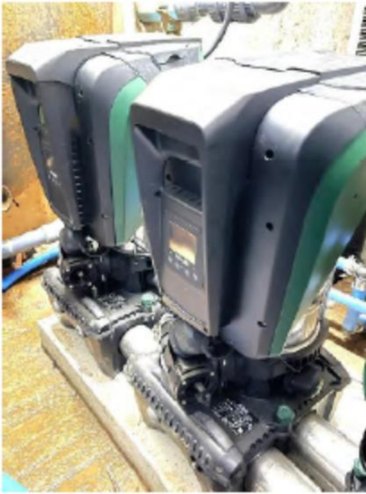
DAB 60/120 VFD, 35 gpm @ 200' TDH each Booster Pumps. Individual Blue Tooth Control Panels Communicate to one another
