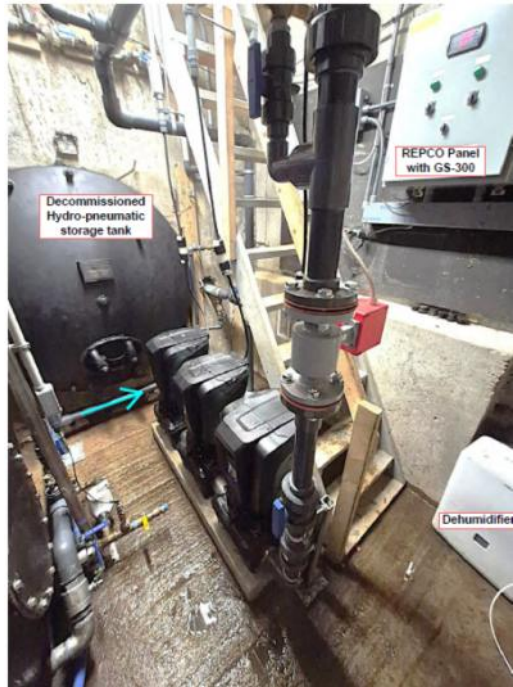
View from End of Pump Room, access Stairs, Pumps, 2" Mag Station Meter & Control Panel
