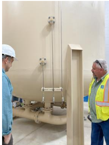
Newly installed PFAS filter at Merrimack Village District water treatment plant, 2020.
