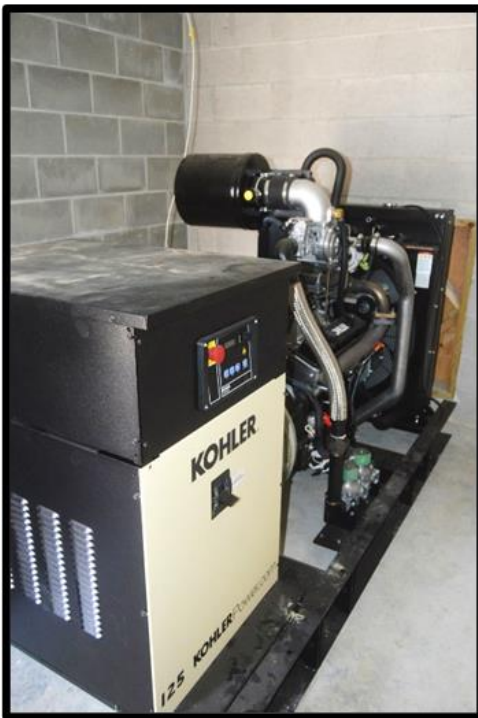
125 KW Standby Gas Generator
