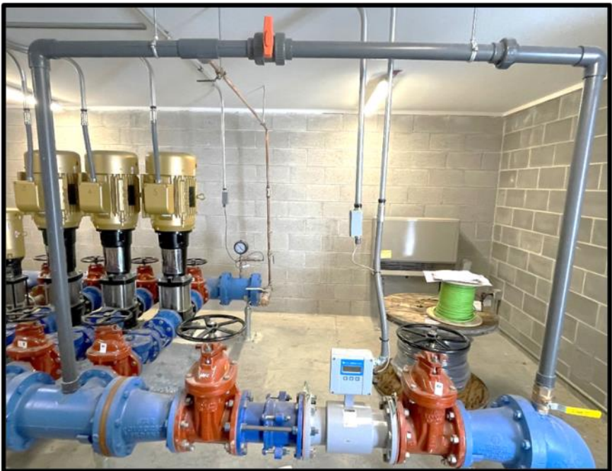
Station 6" Badger M2000 Mag. Meter with 2" Bypass
