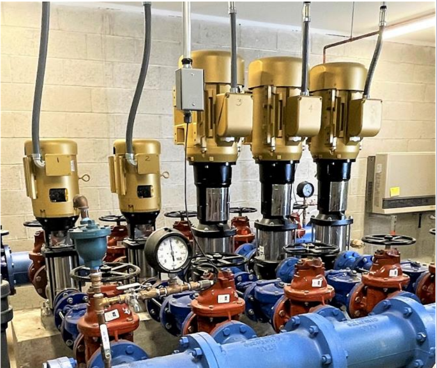
New pumps at the Bowman Place station, Bedford, NH.
