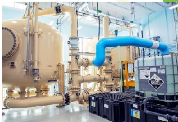
Grove Pond Water Treatment Plant, Ayer, MA (above). 1970s CDM Smith laboratory (below).
