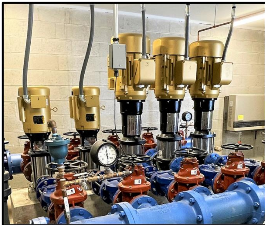
Station Pumps 2@10 H.P. & 3@30 H.P.
