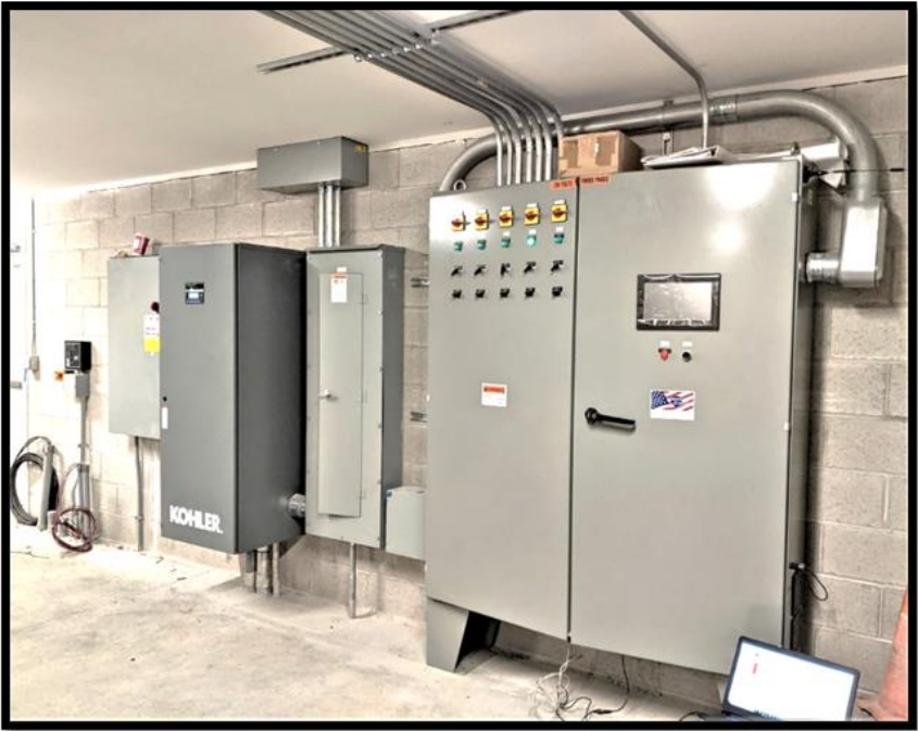
Generator ATS, Electrical Controls and Automatic Control Panel
