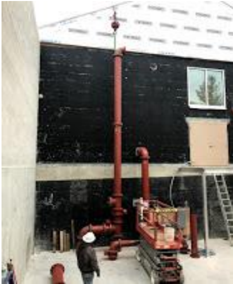
Figure 7-Inside Well 7/8 PFAS WTP Addition
