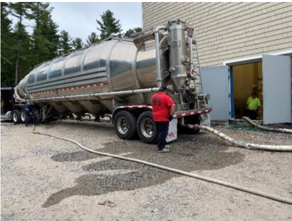
Figure 3-GAC Media Installa- tion-Well 4/5 WTP
