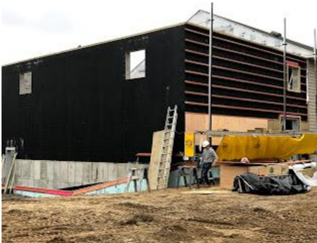
Figure 8- Exterior of Well 7/8 PFAS WTP Addition
