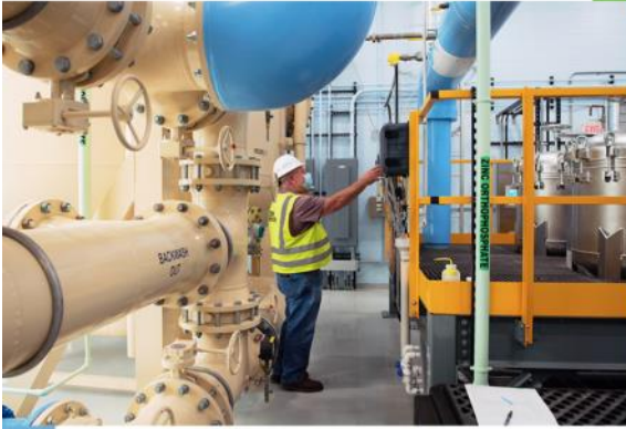
Grove Pond Water Treatment Plant, Ayer, MA
