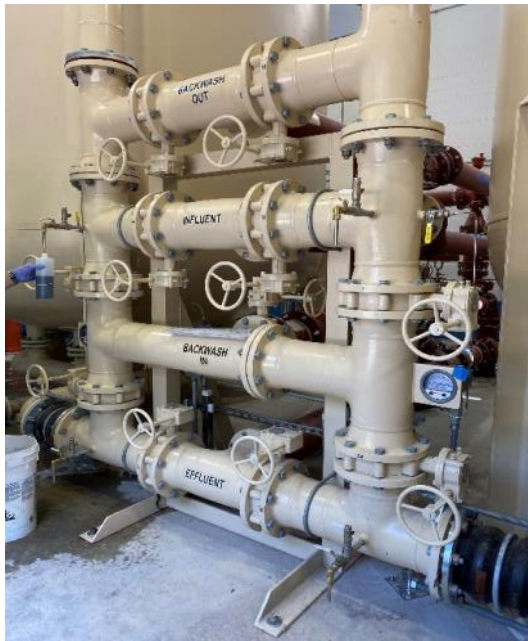
Figure 5-GAC Vessel Pipe Rack & Sample Taps- Well 4/5 WTP
